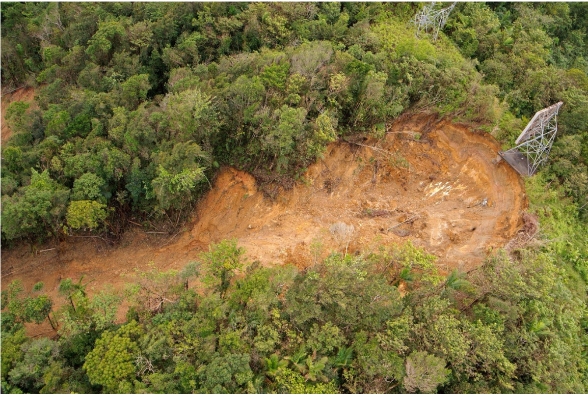
Microwave tower foundation breach by landslide
