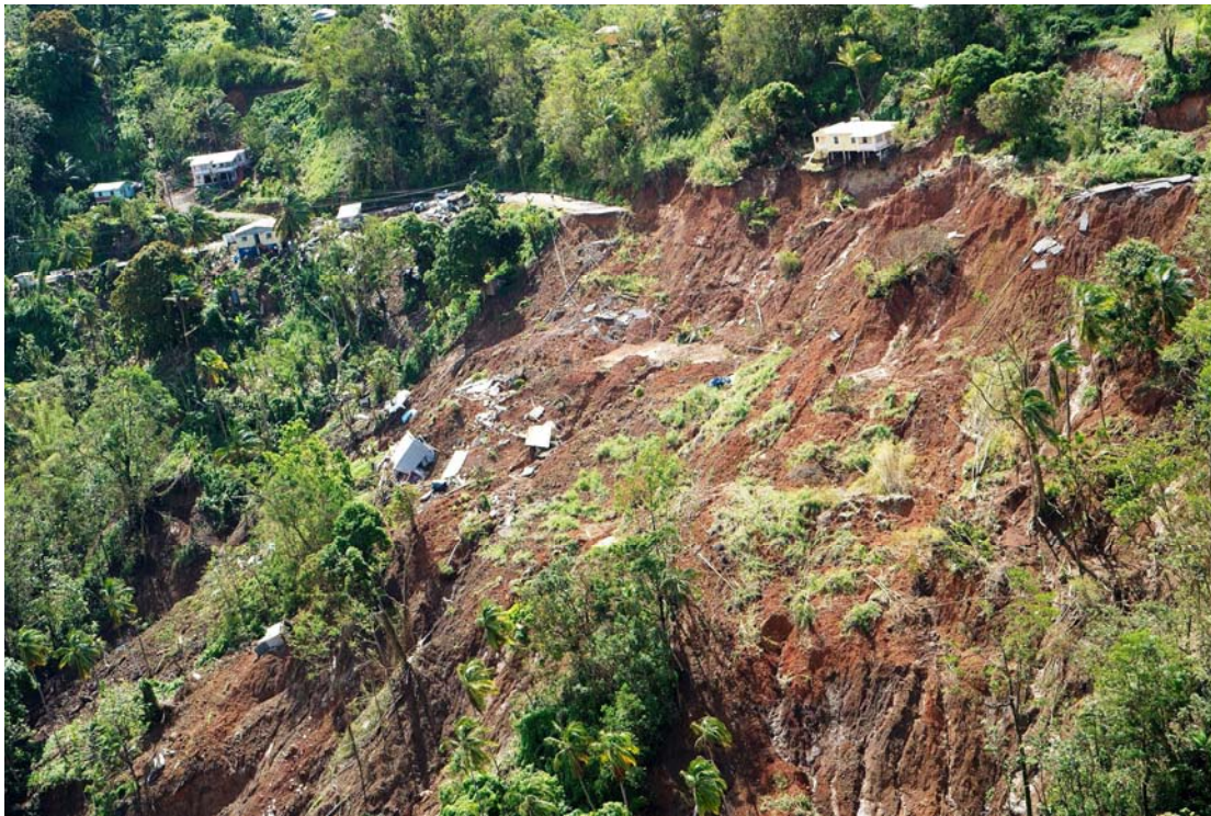
Guesneau: 150 m of roadway in front of yellow house breached by landslide-II
