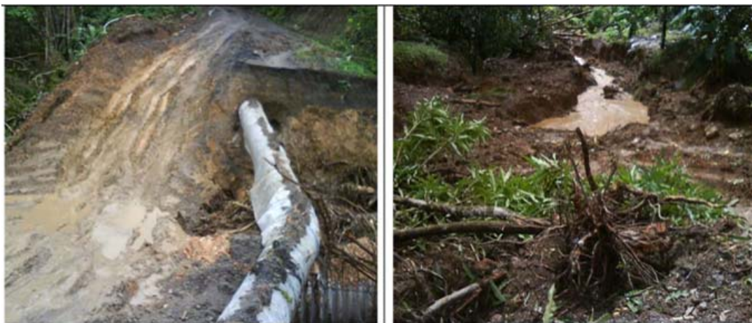
Photo 1b: Damage to access road
