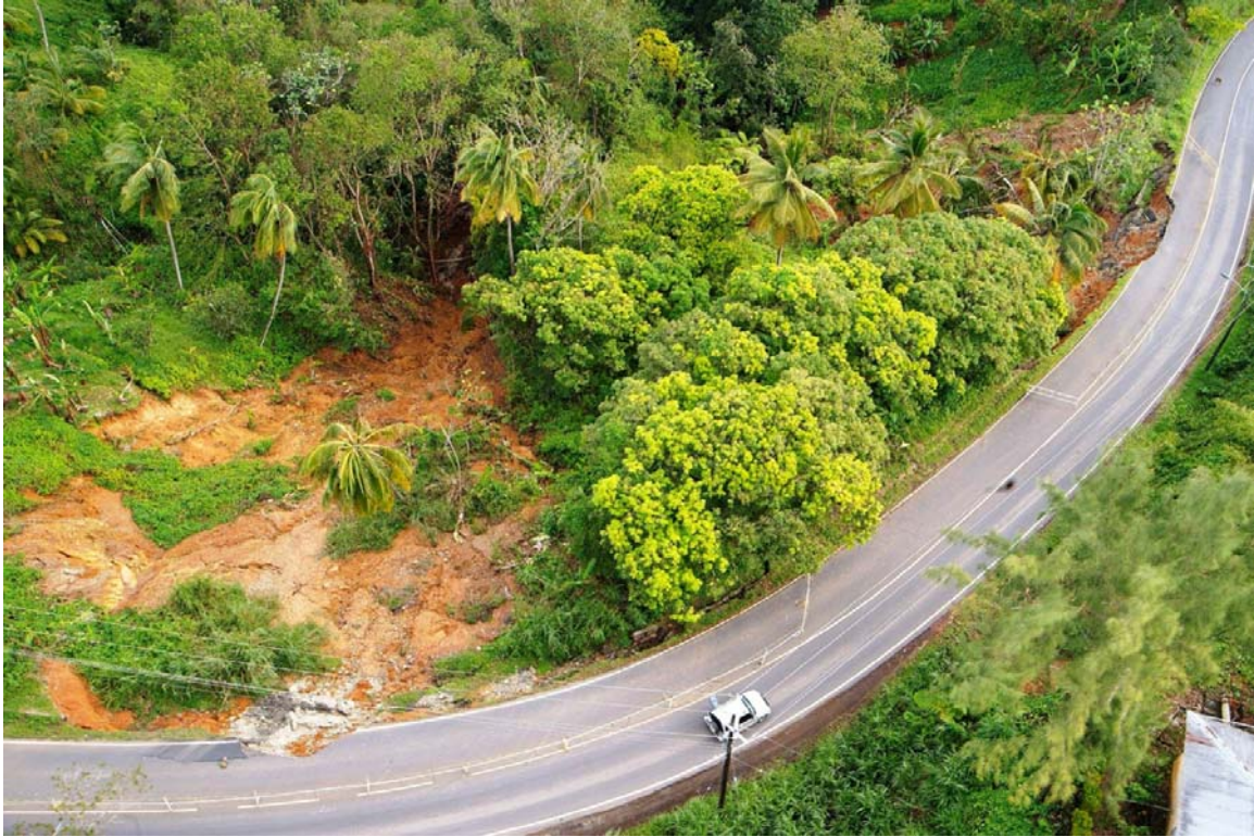
Thomazo, edge failures in roadway, surface runoff related slips
