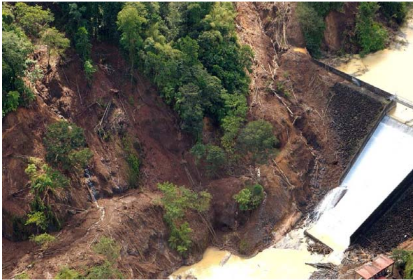
Photo 1a: Damage to spillway
