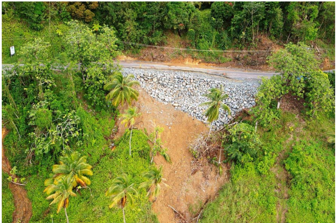
Thomazo, roadway lane failure with boulder pack repair
