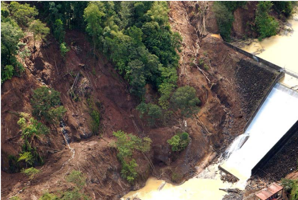
Roseau Dam, minor spillway damage, east abutment
