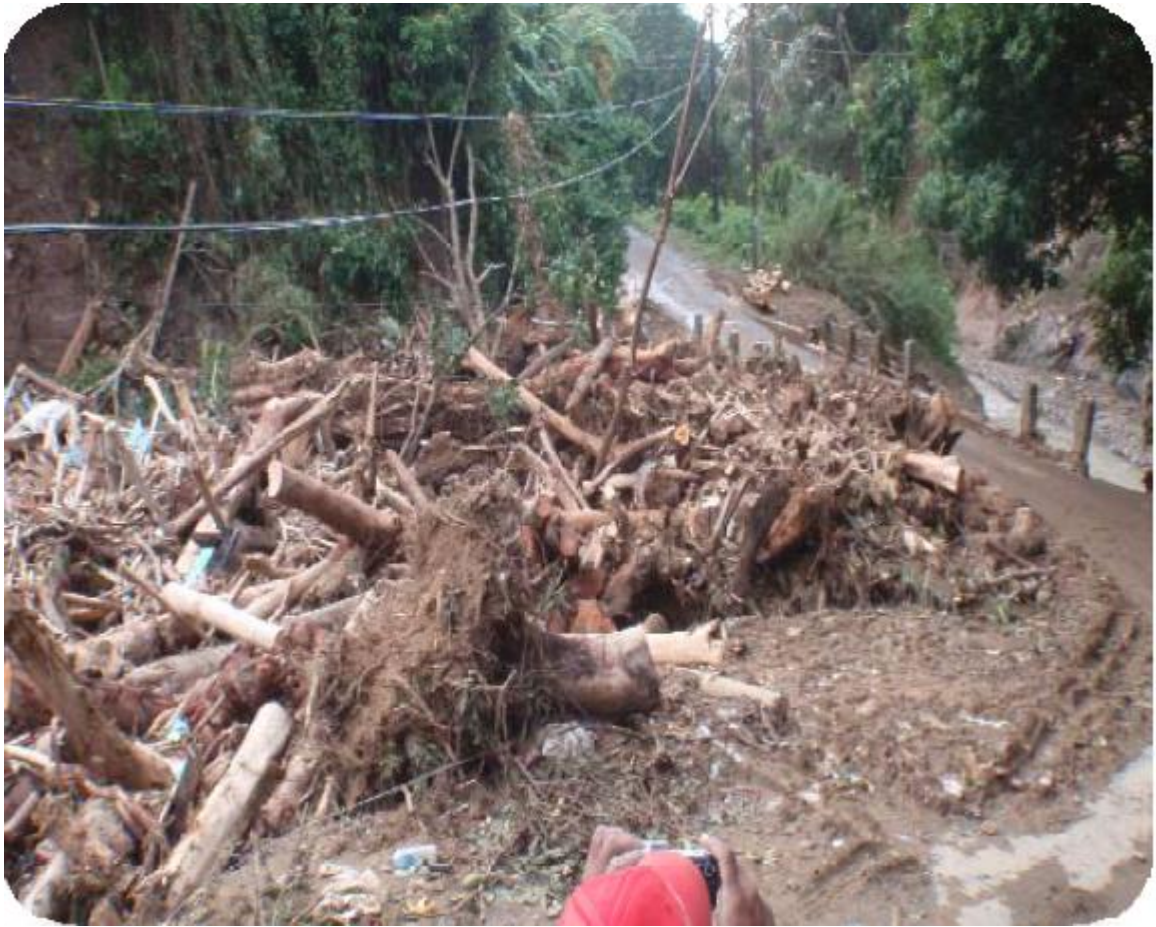
Figure 29 : photographs of Fond Saint Jacques downstream bridge (Mochas' bridge) just after Tomas and after cleaning
