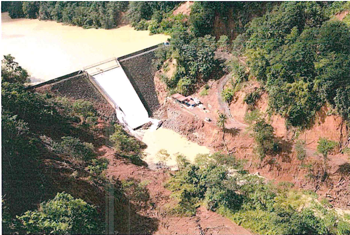
Figure 29: Pump House Conditions after Hurricane Tomas (Macro Socio-Economic and Environmental Assessment of the Damage and Losses Caused by Hurricane Tomas: A Geo-environmental Disaster" February 2011).
